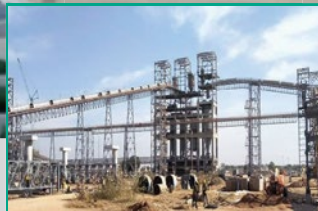
M/s. Ambuja Cements Ltd. AFR Handling System Tonnage: 1400 MT
