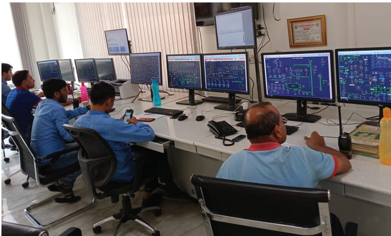
FLSmidth ECS/ControlCenter™ v8 now runs both production lines at Arghakhanchi Cement from a common control room.
