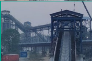
M/s. Dalmia Bharat Cement Ltd. Limestone Handling System Tonnage: 500 MT
