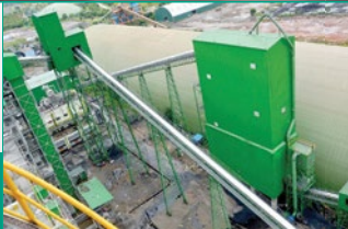
M/s. Nuvoco Vistas Corp. Ltd. Coal & Limestone Handling System Tonnage: 1100 MT
